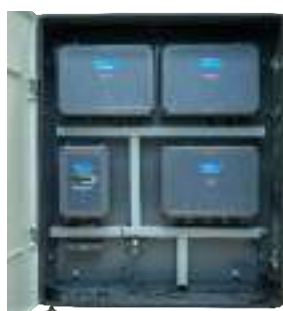
Interior View of xMasm10 - Wired Solution
