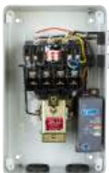
Interior View of MK1.i
