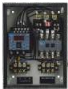
Interior View of MD Starter+ DOL Starter
