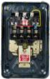
Interior View of MK1 DOL
